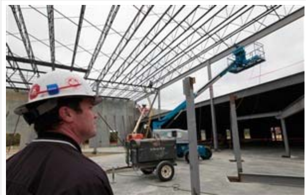
Joey Woodard of general contractor Montgomery Martin Contractors LLC supervises construction of the 37,000-square-foot Living Hope Church at 345 Keough Drive in Piperton. (Photo: Lance Murphey)
